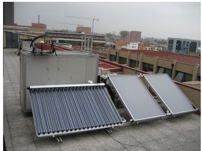
Fig. 1. Collectors installed in the test apparatus.
