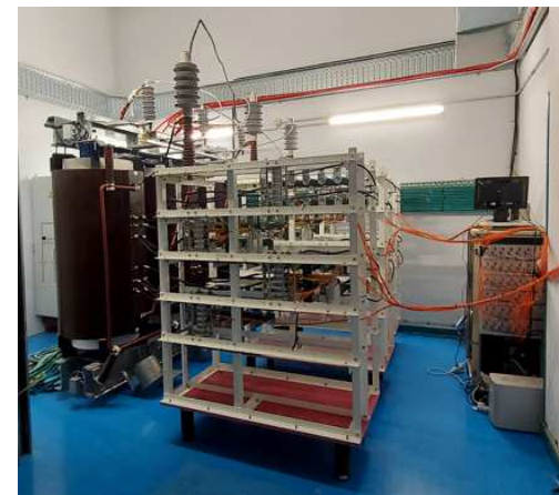
A fully programmable voltage ride-through generator of 3MVA
