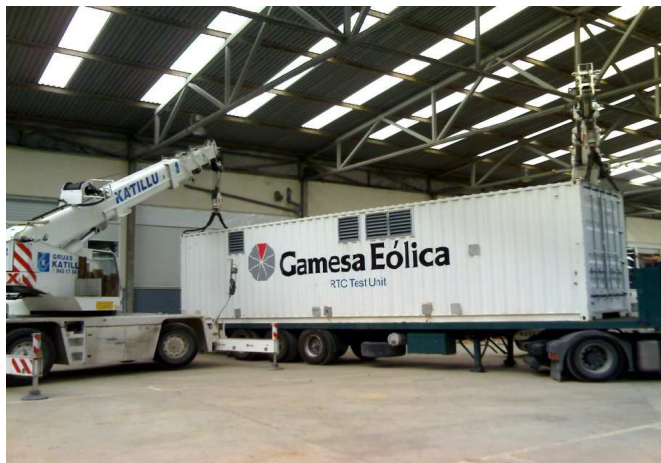
2MVA low voltage ride-through equipment
