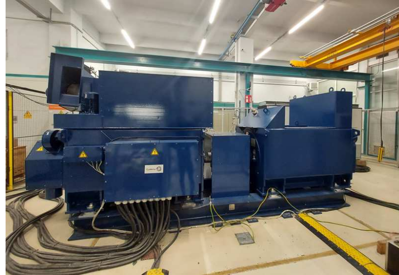
2 MVA drive system
