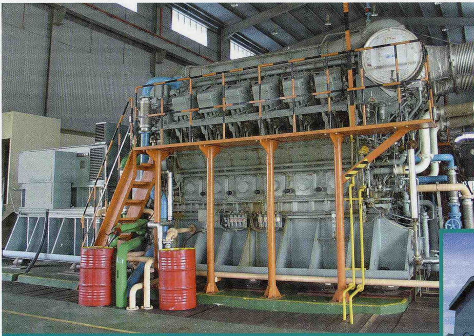
SARAWAK ELECTRICITY SUPPLY CORPORATION 12DK-32B 3500kW×1
