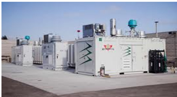
Figure 6-1. Commercial Fuel Cell for CHP Application
