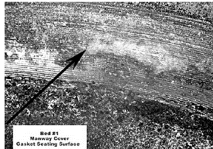
Figure B.33—Corrosion on Gasket Seating Surface
