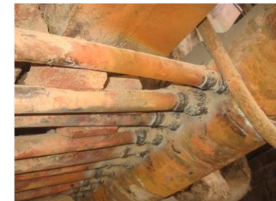
Case study 2- Photo 7-Failures of weld joint of dissimilar materials caused by high steam temperature
