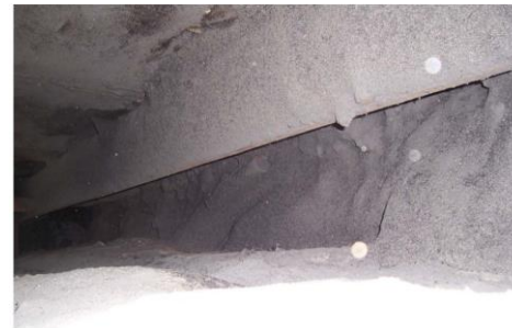
Case study 3- Photo 8: Fuel & ash leakage in the roof
