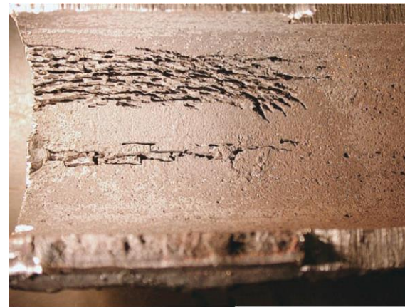
Figure 11.17. Numerous deep, irregularly shaped, discontinuous grooves on the cold-side internal surface of a wall tube
