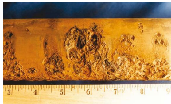
Figure 9.12. Oxygen pitting on the external surface of fire tube.
