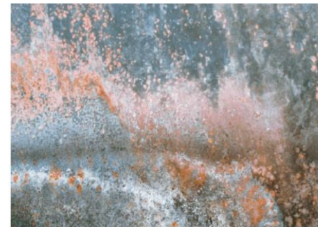
Figure 9.3. Metal loss and red iron oxide layer formation above waterline in steam drum.
