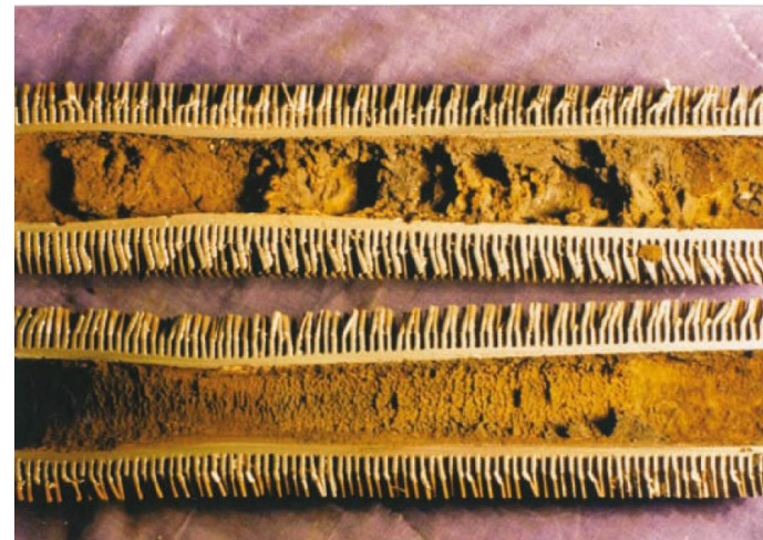
Figure 1.26. Very thick, stratified layers of deposits that covered the internal surface only within a 9" long segment at the location of the failure. Up to \frac{3}{4} of the cross-sectional area was occluded.
