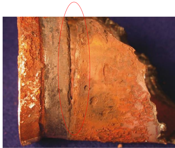
Figure 11.10. Rolled end of a firetube, with a narrow groove immediately adjacent to the location of the tubesheet.
