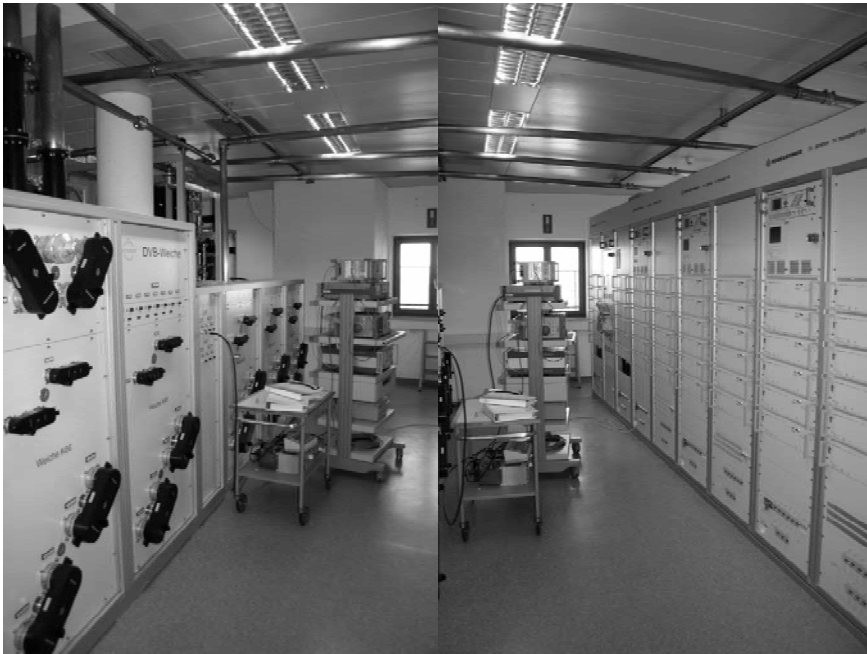
Fig. 31.18. Wendelstein transmitter hall; antenna combiner (left) and UHF transmitters (right)
