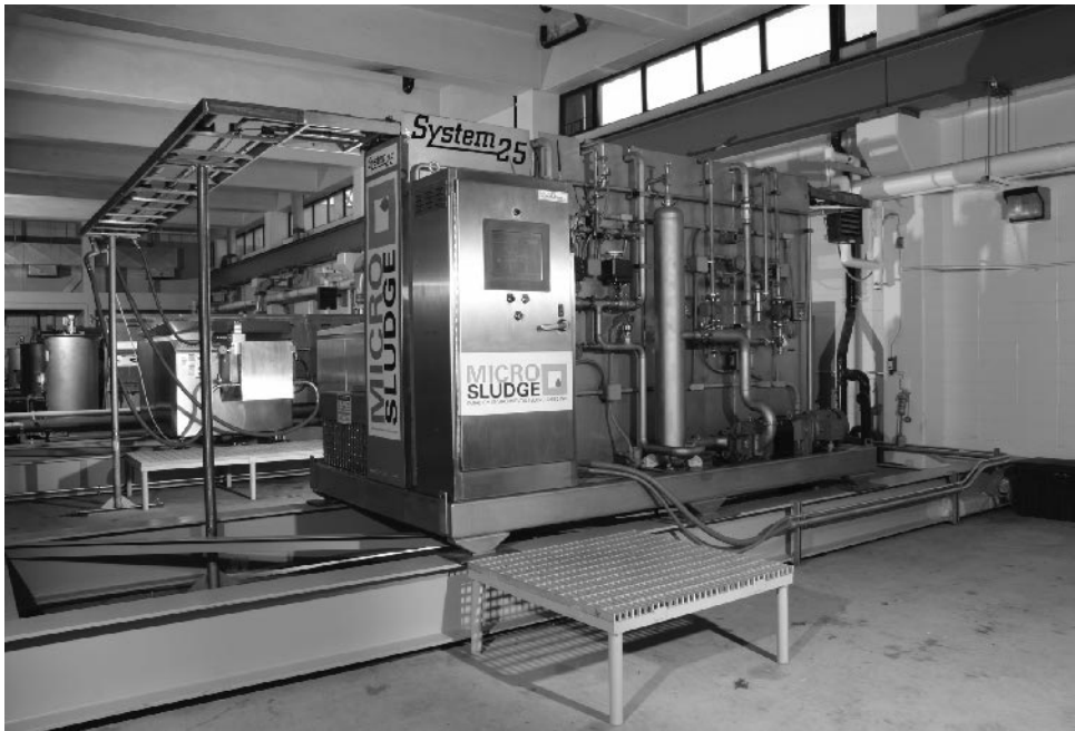
FIG. 11.7. Full-scale MicroSludge system. Source: Courtesy of MicroSludge.
