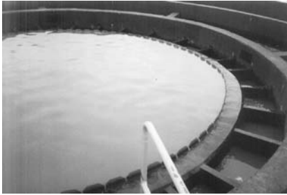
Figure 5.16. Influent distribution structure in a circular reactor (source: Nova Vista WWTP, SAAE Itabira, Minas Gerais, Brazil)
