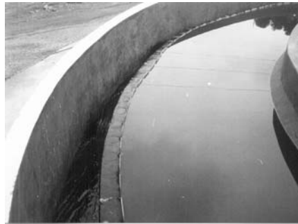
Figure 5.19. Effluent collection device (plate with V-notch weirs) Source: Nova Vista WWTP, Itabira, Minas Gerais, Brazil
