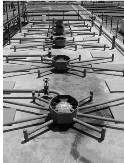
Figure 5.17. Influent distribution structure in a rectangular reactor (source: Ipatinga WWTP, COPASA, Brazil)
