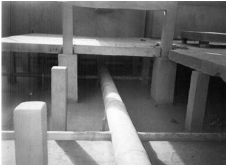
Figure 5.5. Sewage distribution device at the bottom of an anaerobic filter (Ipatinga WWTP, COPASA, Brazil)
