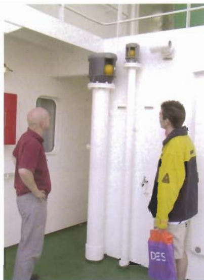
Raised tank vents
