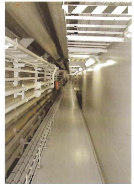
Cable trays and pipes in the corridor between the forward and aft engine room of a stone-dumping vessel
