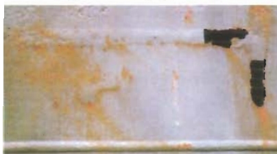
If the mill scale is not properly removed, it will eventually let go
