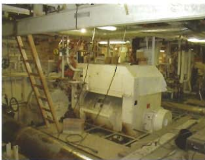
Main-engine driven generator
