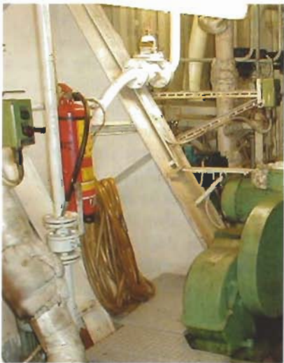
Small bilge pump of the bilge-water separator
