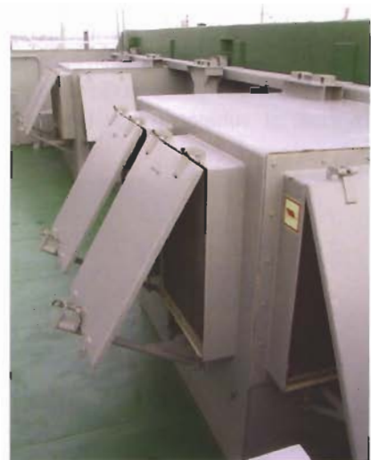
Ventilation grill with cover
