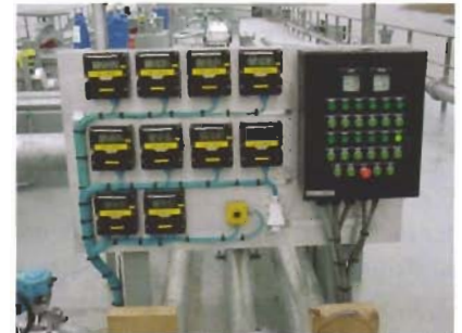
Detail of cargo-deck. Electrical control and monitoring equipment. The tank-level indication system with the blue cables is executed in intrinsically safe technology and the pump controls on the right in explosion-proof execution.
