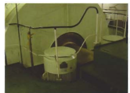
Main engine flywheel with intermediate shaft and main lubricating-oil pumps, electric motors
