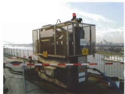
Water resistance to load test of generators
