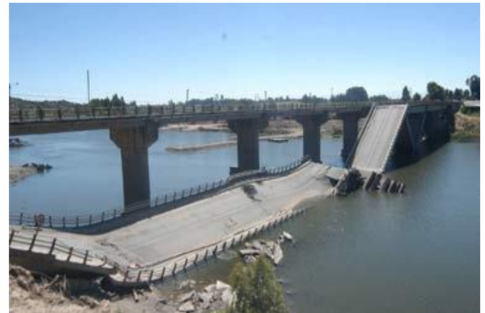
Figure 2 . Loncomilla Bridge collapsed due to scour. (Fisco deberá pagar. 2011)
