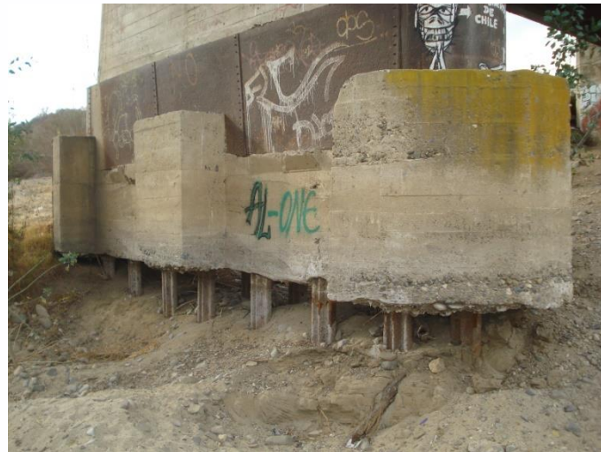
Figure 1. Eroded soil around the pier of the Curacavi Bridge, in Metropolitan Region, Chile.
