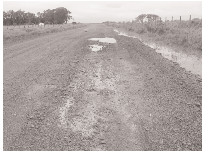
FIGURE 3 Pavement condition in July 2007 where test section was built.
