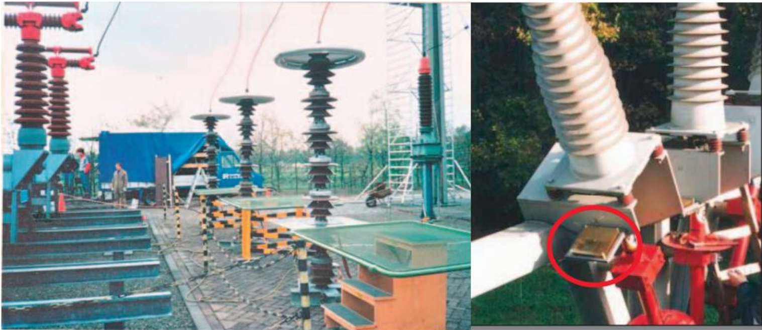
Fig. 1. Practical constructions of sensors, left: “improvised” metal plates near switch gear; right: specially developed sensor (within circle) near cable termination
