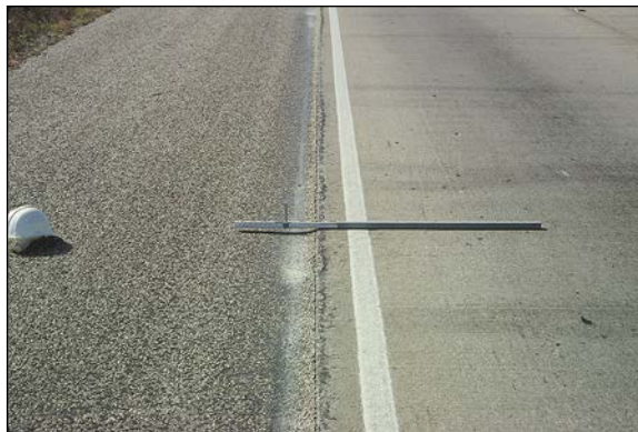
FIGURE 115 Distress Type CRCP 9—Lane-to-Shoulder Dropoff.
