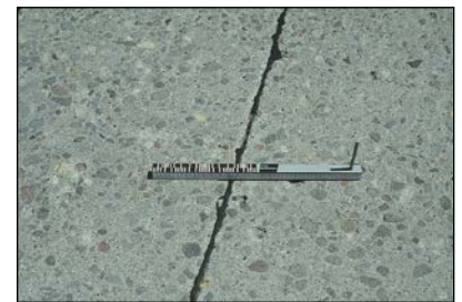
FIGURE 62 Distress Type JCP 5—Moderate Severity Joint Seal Damage.
