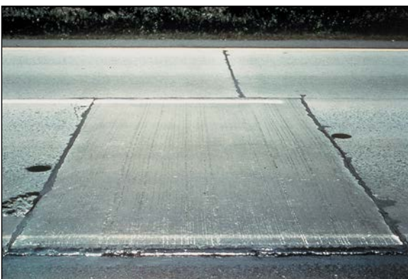
FIGURE 88 Distress Type JCP 15—Large, Low Severity PCC Patch.
