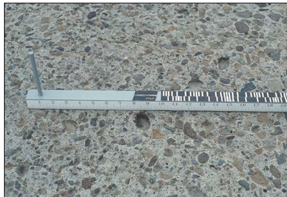
FIGURE 105 Distress Type CRCP 6—Popouts.
