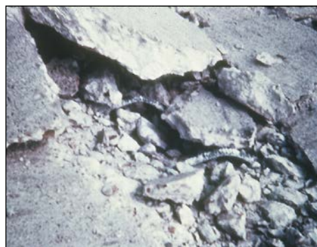
FIGURE 109 Distress Type CRCP 7—Exposed Steel in a Blowup.
