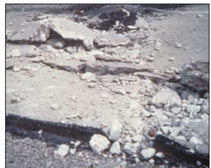
FIGURE 108 Distress Type CRCP 7—Close-up View of a Blowup.
