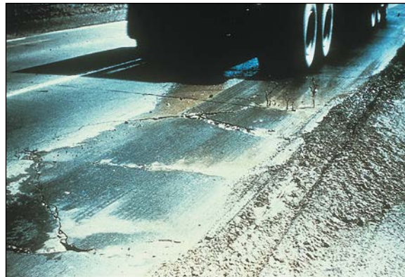
FIGURE 89 Distress Type JCP 16—Water Bleeding and Pumping.
