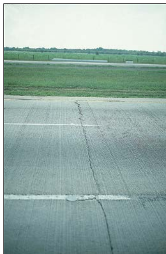
FIGURE 112 Distress Type CRCP 8— Moderate Severity Transverse Construction Joint Deterioration.
