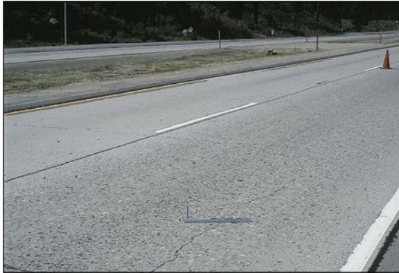
FIGURE 55 Distress Type JCP 3—Low Severity Longitudinal Cracking.
