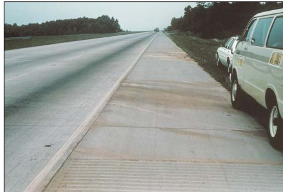
FIGURE 131 Distress Type CRCP 14—Water Bleeding and Pumping.
