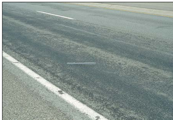
FIGURE 37 Distress Type ACP 11—Loss of Texture.
