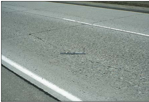
FIGURE 56 Distress Type JCP 3—Moderate Severity Longitudinal Cracking.
