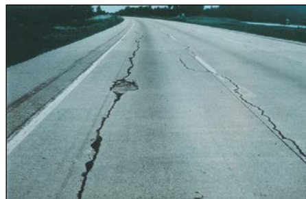
FIGURE 95 Distress Type CRCP 2—High Severity Longitudinal Cracking.
