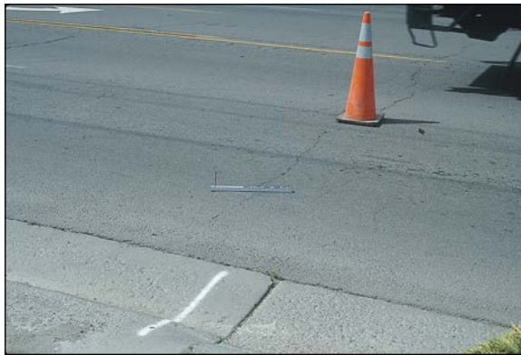
FIGURE 20 Distress Type ACP 6—Moderate Severity Transverse Cracking.
