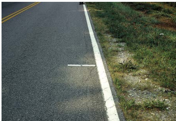
FIGURE 12 Distress Type ACP 3—Low Severity Edge Cracking.
