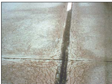
FIGURE 52 Distress Type JCP 2—Moderate Severity “D” Cracking with Well-Defined Pattern.
