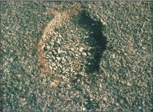
FIGURE 29 Distress Type ACP 8—Moderate Severity Pothole, Close-up View.
