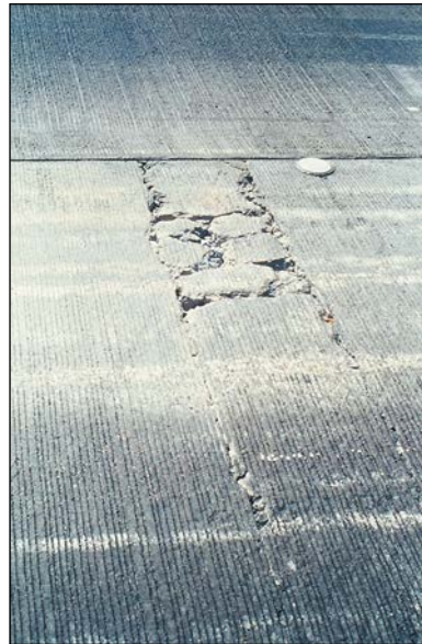
FIGURE 126 Distress Type CRCP 12—High Severity Punchouts.
