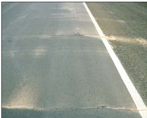
FIGURE 46 Distress Type ACP 15—Fine Material Left on Surface by Water Bleeding and Pumping.
