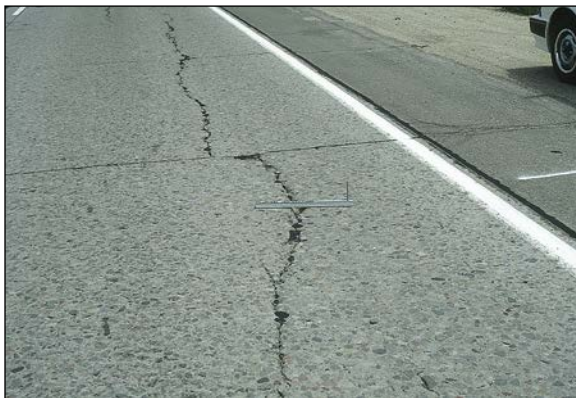
FIGURE 57 Distress Type JCP 3—High Severity Longitudinal Cracking.
