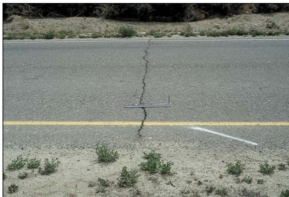
FIGURE 21 Distress Type ACP 6—High Severity Transverse Cracking.
