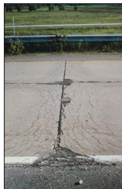
FIGURE 53 Distress Type JCP 2—High Severity “D” Cracking with Loose and Missing Material.
