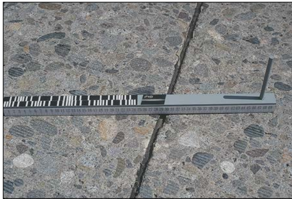
FIGURE 133 Distress Type CRCP 15—Longitudinal Joint Seal Damage.
