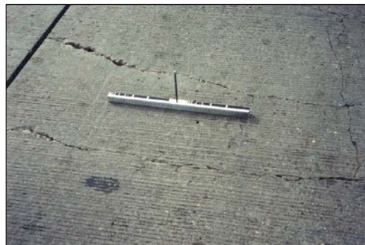
FIGURE 124 Distress Type CRCP 12—Low Severity Punchout.
